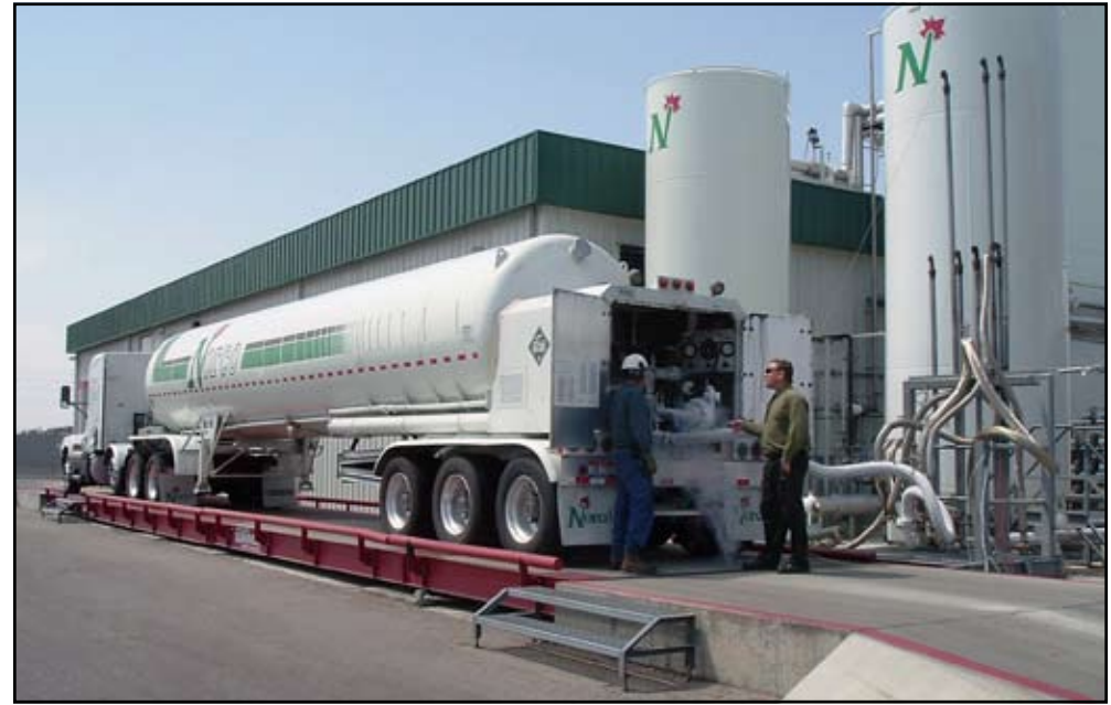
Howard Briggs, right, air separation plant manager for Norco, Inc. in Nampa, Idaho, helps Sean Welch, senior plant operator, fill a liquid nitrogen trailer. Norco's new plant, to be built in Moses Lake, Wash., will serve as the distribution center for up to 20 long-haul truck drivers.
